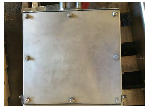
Bolted Covers Restrict Access to Only Qualified Maintenance Personnel
